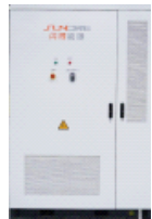
215kWh储能 215kWh energy storage
